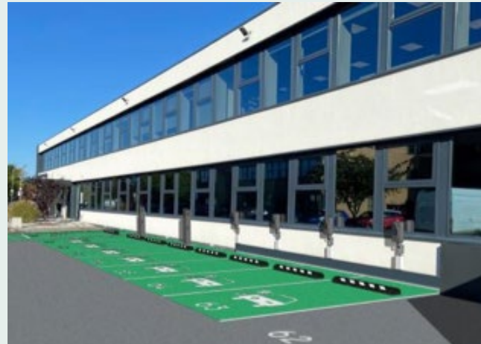
8x22kW Etrell EV sockets
