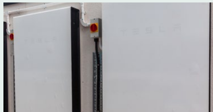
40kW of battery storage
